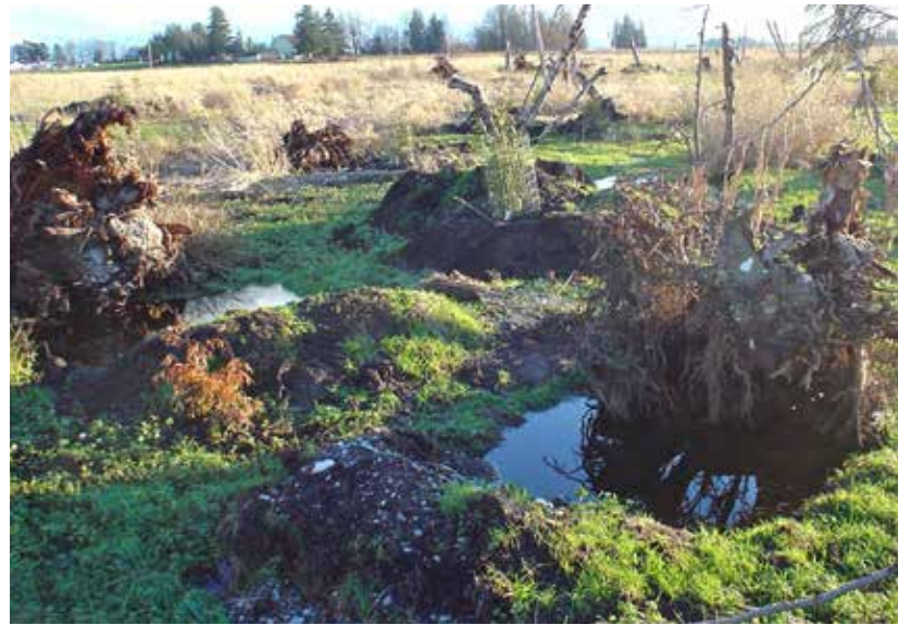
Small pits and mounds were dug by an excavator as it placed large woody debris in this project.
